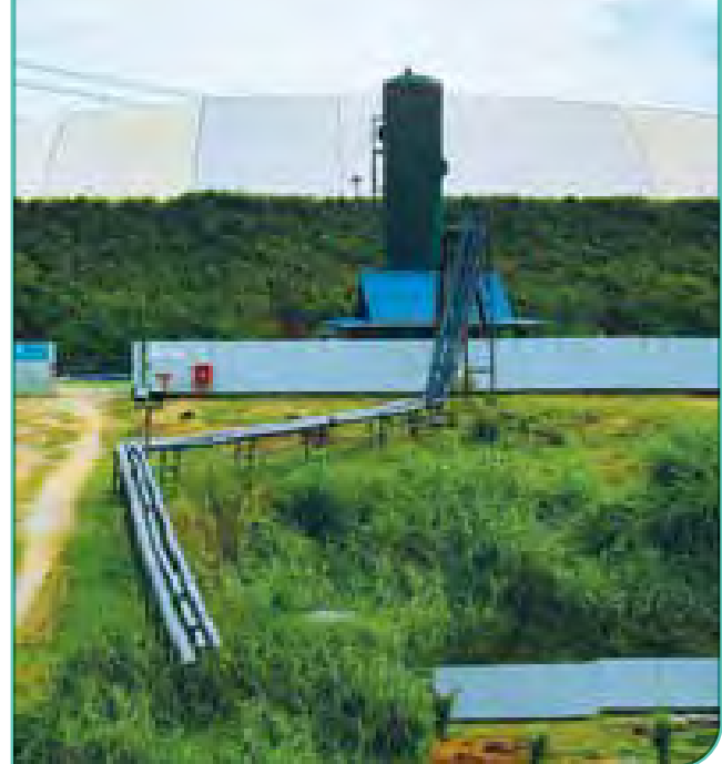
Biogas plant at Telok Sengat Palm Oil Mill, Kota Tinggi, Johor
